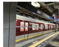
Platform edge gates with cables (Platform 2 at Tsuruhashi Station)
