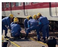
Drill to put a derailed car back onto the tracks (accident/disaster recovery drill)
