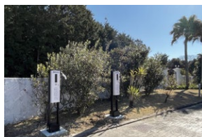
EV chargers (Miyako Resort Shima Bayside Terrace)
