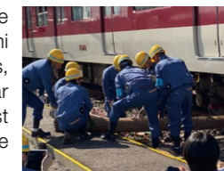
Drill to put a derailed car back onto the tracks (accident/disaster recovery drill)
