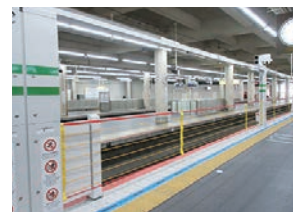
Fitted movable platform edge gates at Osaka-Abenobashi Station
