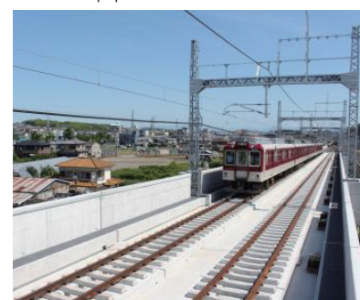
Grade separation work between Kishi Station and Tondabayashi Station on the Nagano Line
